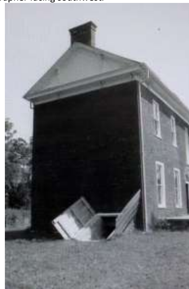
7 of 29: West elevation, showing brick chimney, fishscale shingles in gable, brackets and open cellar doors; Photographer facing northeast.
