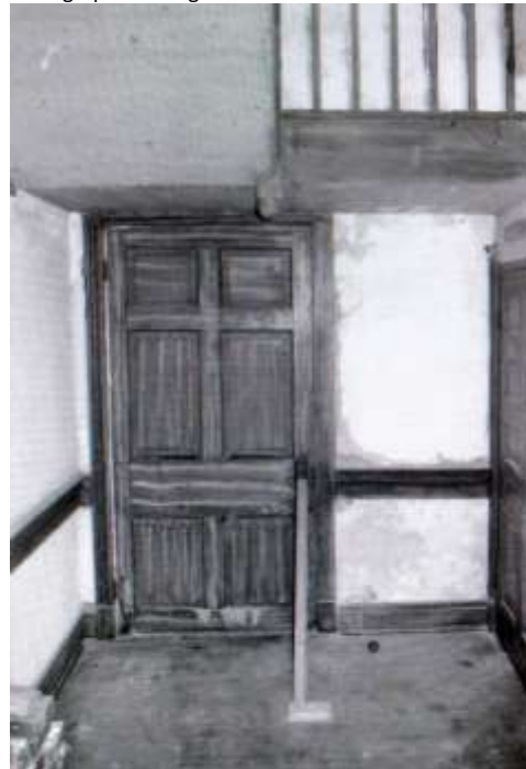
11 of 29: Rear exit door taken from entrance hall, showing wood graining on paneled doors and molding; Photographer facing north.
