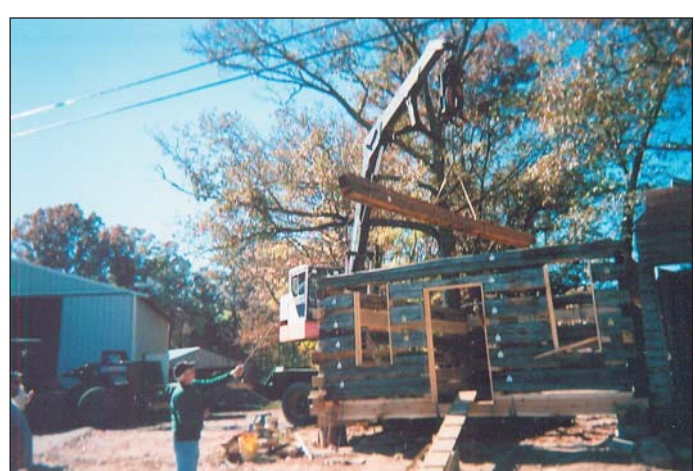
After the knuckle boom peeled away the roof and rafters, workmen used it to lift each log off and away from the structure.
