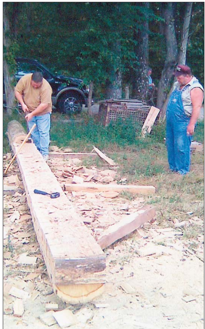
Some of the original hand-hewn logs had to be completely recreated. Here, Joel Keeton and Paul Keeton work to square a log in order to replace one that was too damaged to be repaired.
